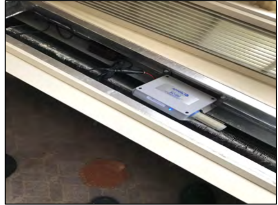
SGFC-400 Installed in Cassette AirCon
