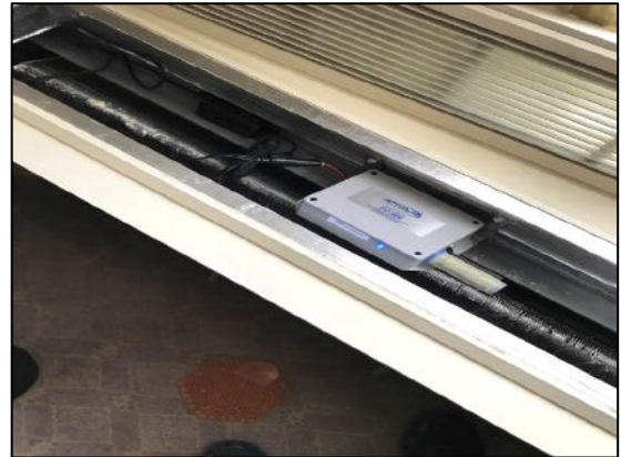
SGFC-400 Installed in Cassette AirCon
